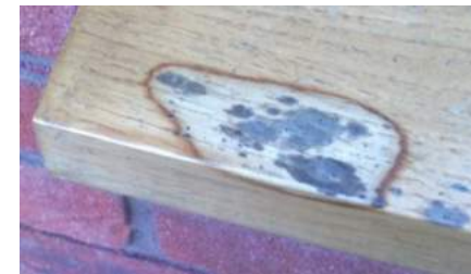
Localised staining can be sanded out using a detail sander and the coating system reinstated
